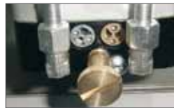
By pass valves
