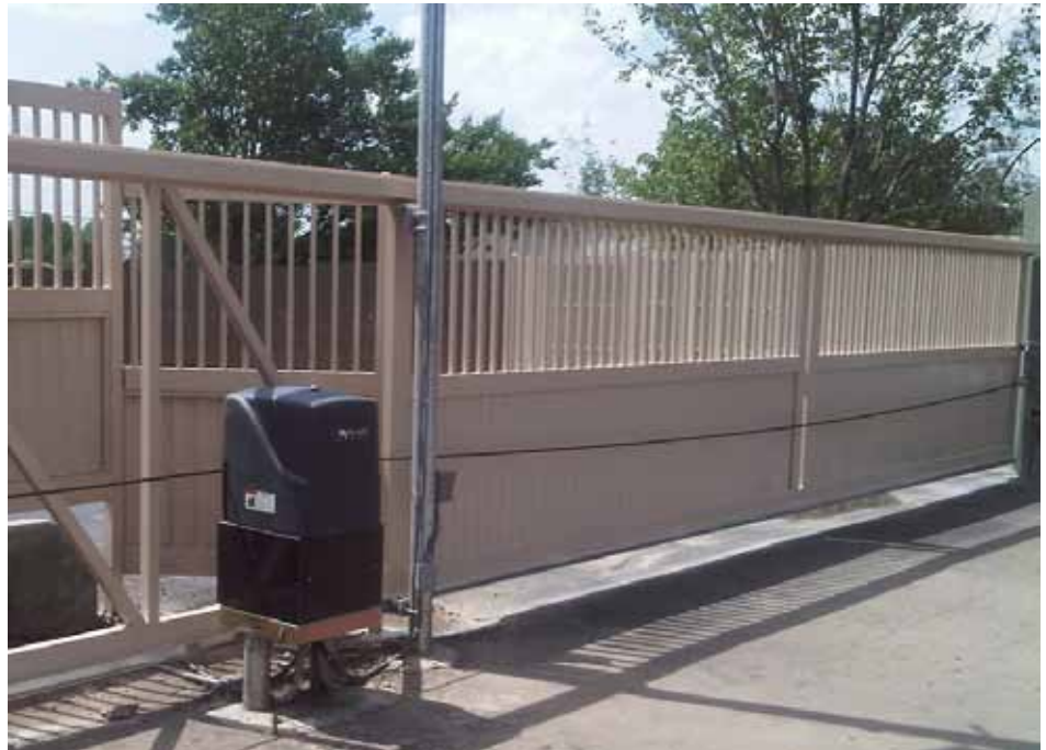
SlideSmart DCS 10F (Solar) installed on base riser that houses two extended 50 Ah batteries for high cycle solar operation. 24V DC solar panels charge the batteries for continuous, reliable operation.
